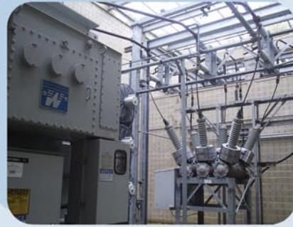
SUBSTATION AND DISTRIBUTION
