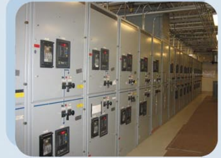
MEDIUM VOLTAGE AND SWITCHGEARS
