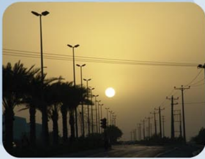
STREET LIGHTING AND TRANSMISSION LINE
