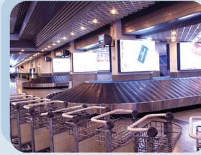
FACILITIES AIRPORT LIGHTING
